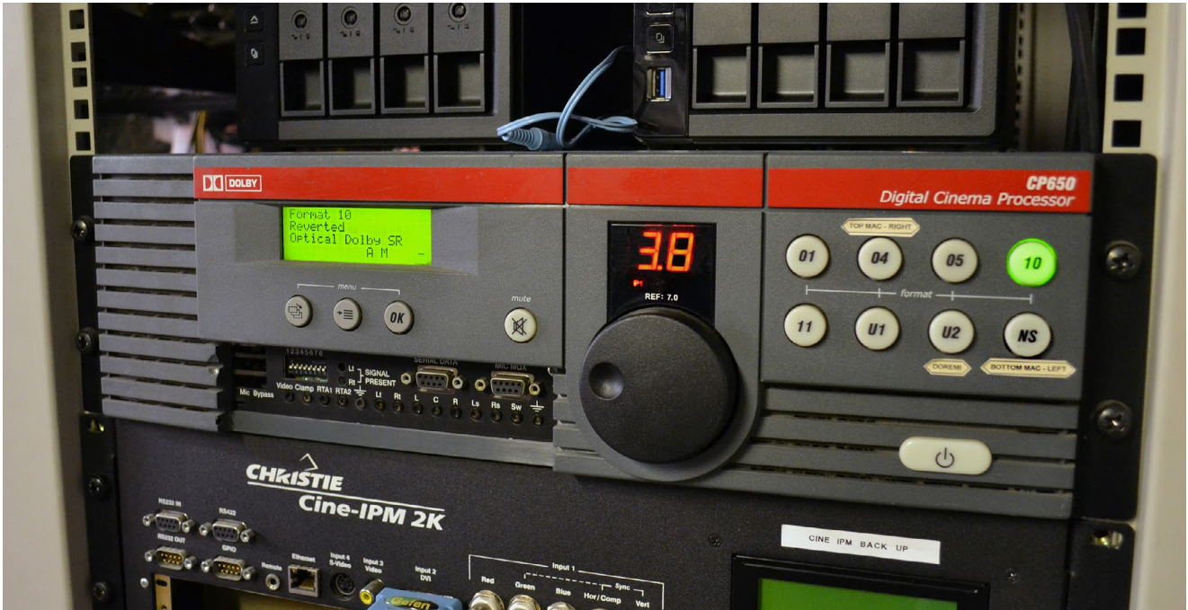
A Dolby CP650 sound processor within an equipment rack
